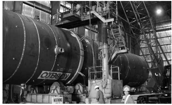
図3 現地工事建屋内での最終溶接 Fig. 3 Welding of final seam inside site fabrication shop
