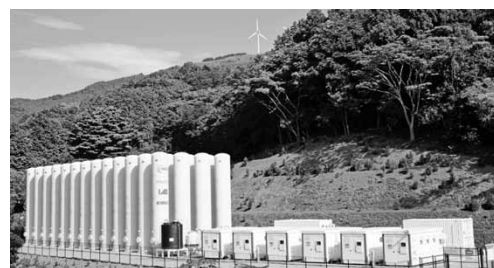
図4 1 MW大型実証設備の外観 Fig.4 Appearance of 1 MW large-scale demonstration plant
