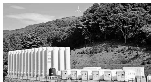
図4 1 MW大型実証設備の外観 Fig.4 Appearance of 1 MW large-scale demonstration plant
